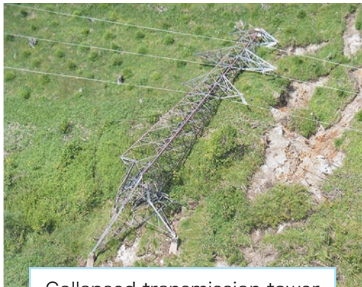
Collapsed transmission tower
