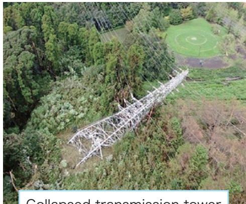
Collapsed transmission tower
