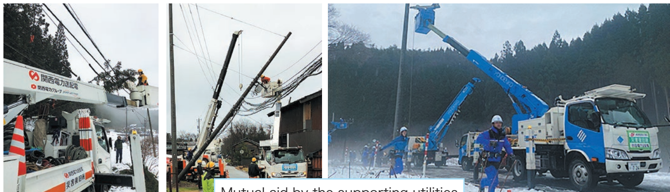
Mutual aid by the supporting utilities
